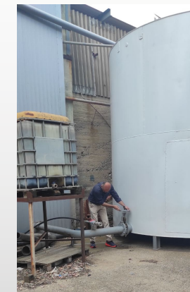
Fire sprinkler water supply line.
