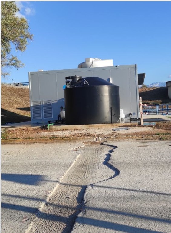
Excavation of an irrigation conduit within the premises of the Athenian Brewery facility.
