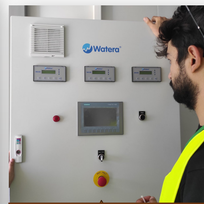
PLC of the system
